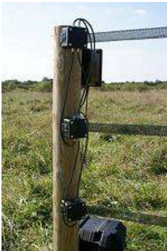
Control Tower Tensioner
