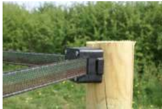
A corner insulator
